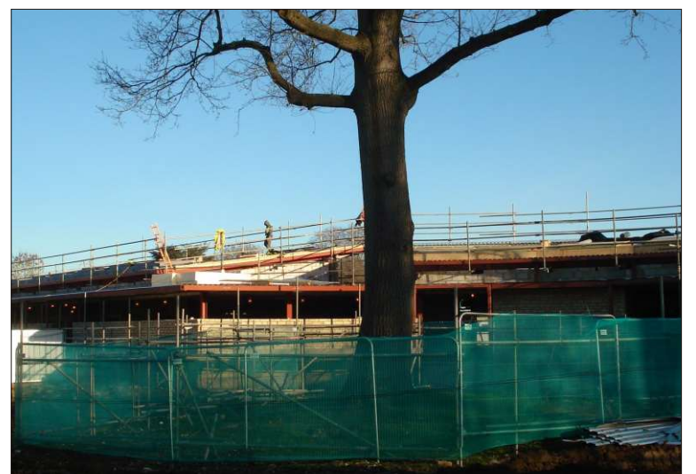
Construction of the new school around an old oak tree. Protective fences erected around the tree. October 2010.
