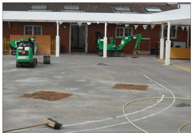
Construct on site - carpets and surfaces protected, workers compound secured, site kept tidy on a daily basis. Appropriate machinery for the job - small enough to drive through the corridors. August 2011
