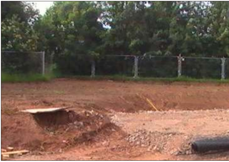
Site appraisal to gauge changes in level and prepare a concept to accommodate the slopes on the site. June 2009
